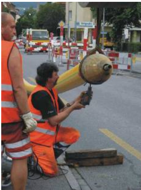
The new HDPE pipe OD 250 mm (10") is pulled in with the expander cone Ø 325 mm (12.8").
