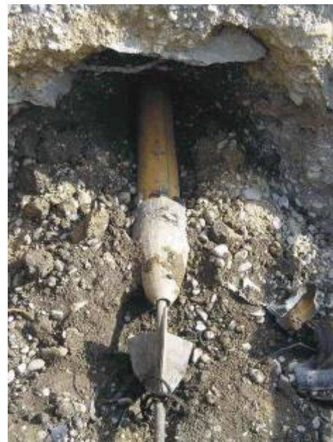
The 3-wing cutter and the new HDPE pipe OD 250 mm (10") reach the intermedium pit.
