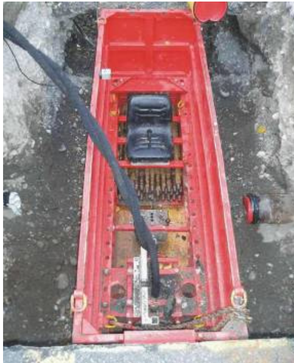
The TERRA-HYDROCRACK HC 600 C+ is positioned in the working pit. The rods are in the magazine underneath the operator seat.
