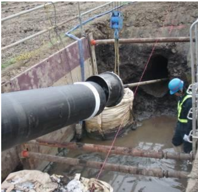
The bore channel is reamed up to \varnothing 800 mm (32"). Now the HDPE pipe OD 560 mm (22") can be pulled in.
