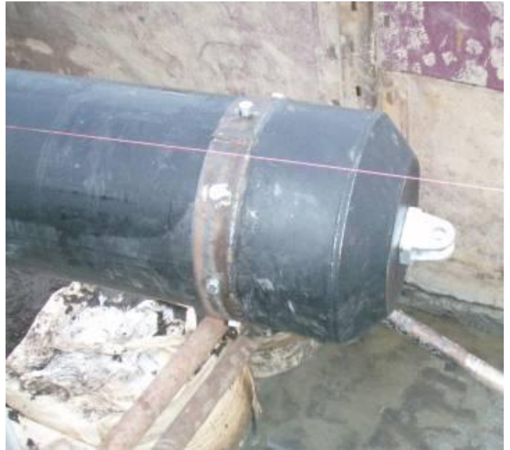
The expander chuck is assembled in front of the HDPE pipe 560 mm (22").
